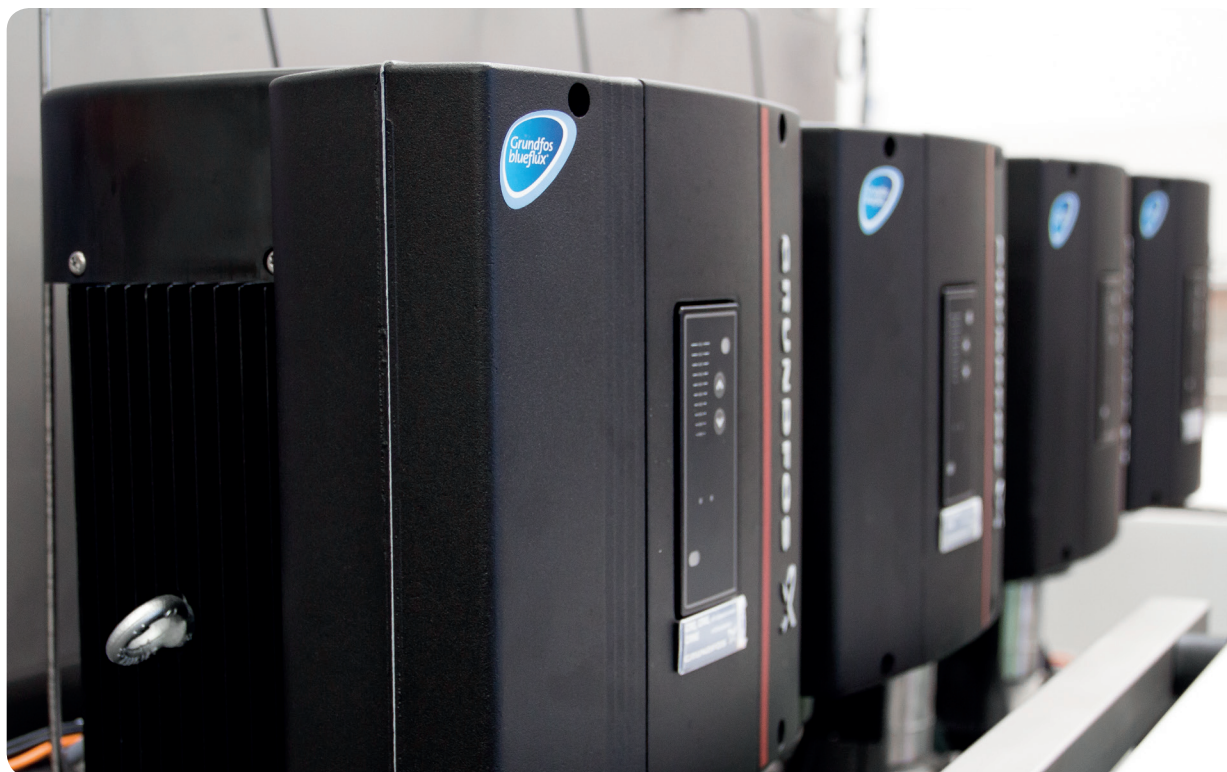
The LDC-Q 400/20 with four 5,5 kW pumps
