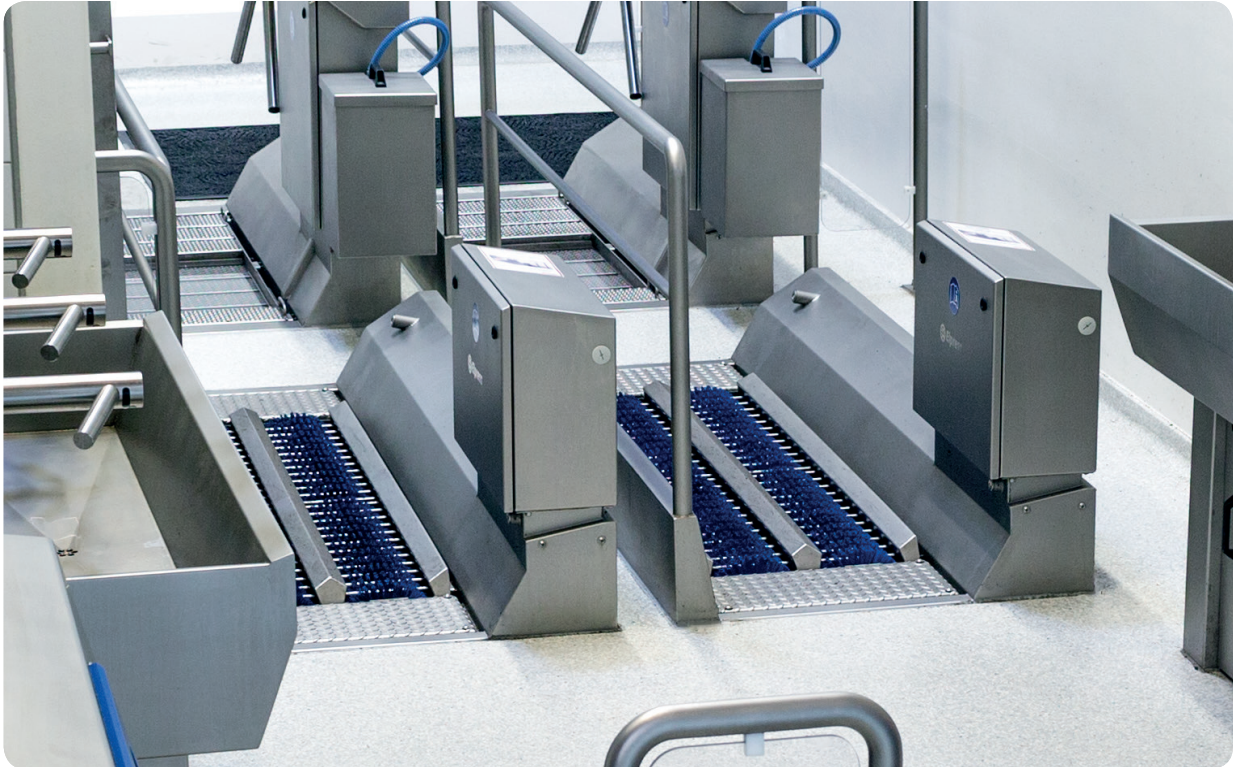
The DZW-1500-R, built in as part of a complete hygienic room.
